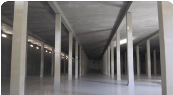
DRINKING WATER TANKS
